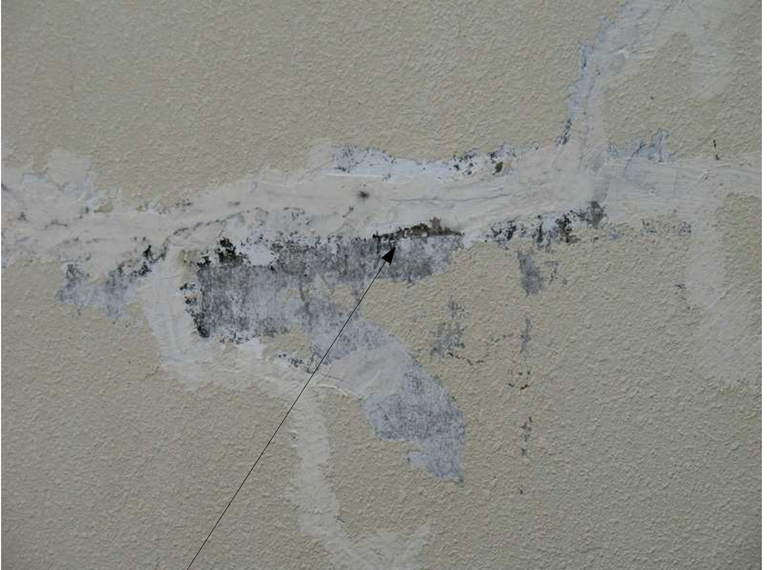
Cracks have been filled with Thioflex filler, and acrylic putty as a finish
