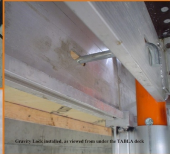
End Filler Beam with Gravity Locks installed (note: Telescopic Beam also installed)
