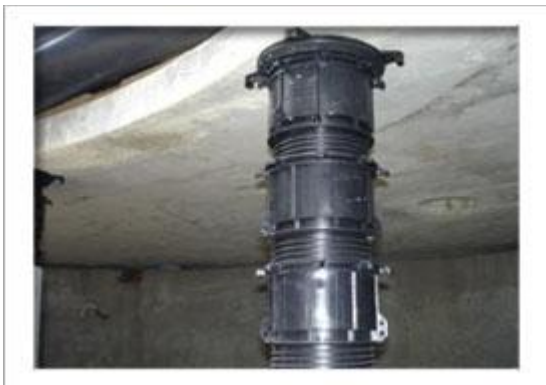
Heavy loads such as pre-cast concrete slabs can be accommodated by VersiJack ® , shown here under concrete slabs at 'Waterplay' in Brisbane, above and the completed installation at right.
